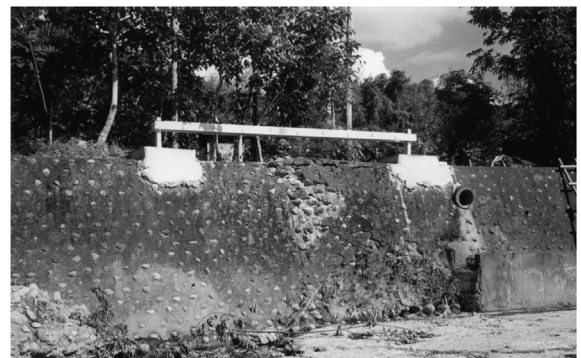
Fig. 2. (a) Schematic representation of our rod-type creepmeter [10] set up across an active fault rupturing a concrete wall. (b) Photograph of creepmeter 4 at Chinyuan.
